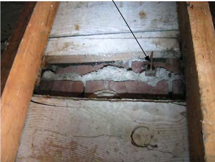
Photo #4 – 1x8 T&G exterior sheathing with brick veneer and evidence of masonry ties
