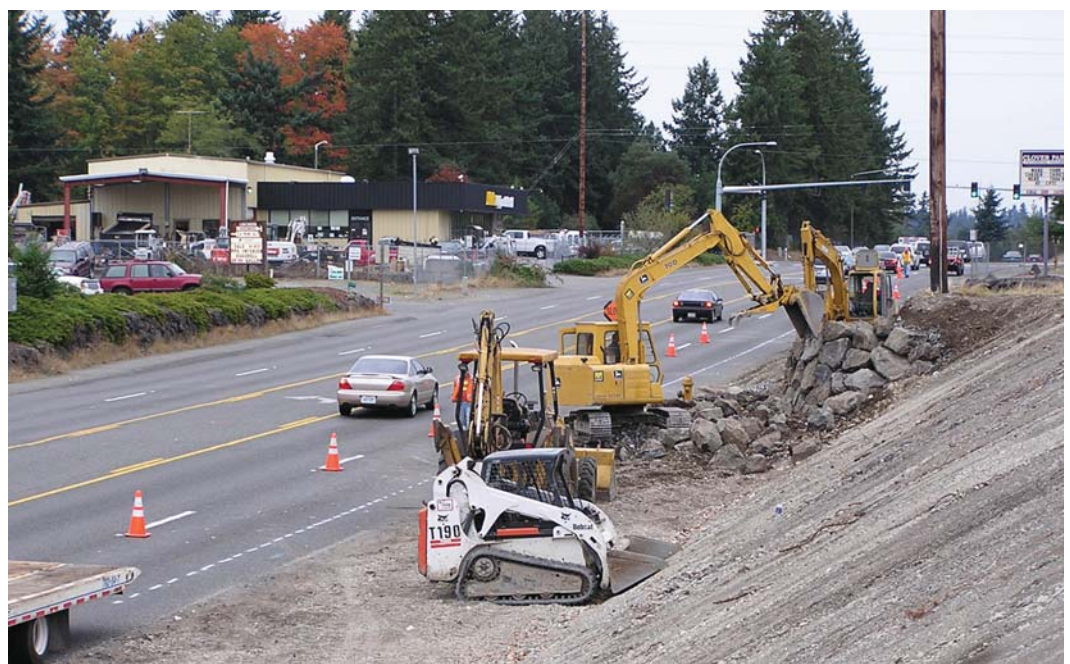
Construction is under way on Steilacoom Blvd. The project will add curbs, gutters, sidewalks, lighting and landscaping and is being paid for by the property owners through a local improvement district.
