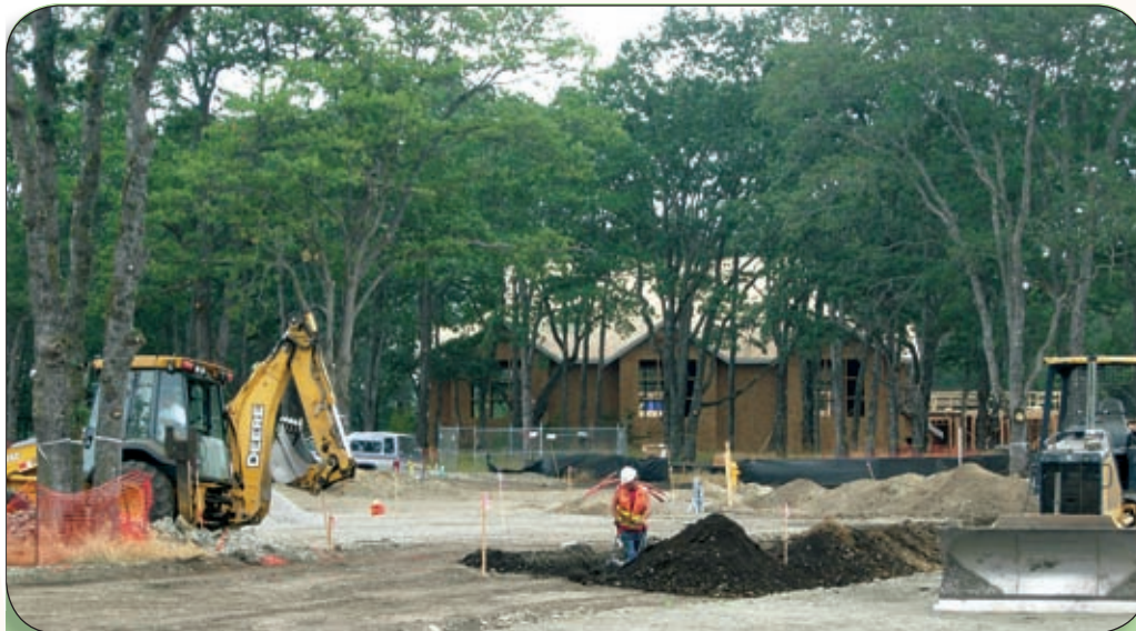
Construction continues at Oak Grove Apartments (corner of Steilacoom Blvd. and Lakewood Dr.). Up to 254 high-end units will be built at Oak Grove and a large number of the beautiful, historic oaks will be preserved. It is one of only a few apartment complexes currently under construction in Western Washington.
